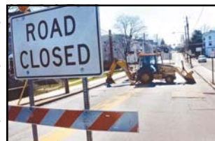
Main Street in Hatfield, PA closed since Thursday, March 24, due to sinkhole.
