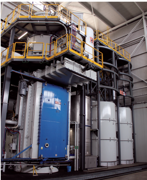
Fig. 1 — The vertical vacuum IQ furnace line.
